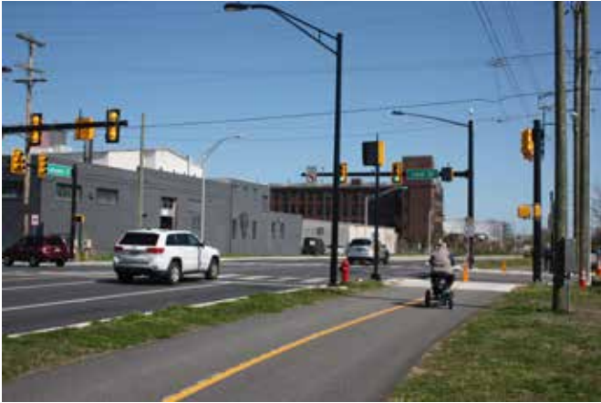
Photo 10: View facing east of new asphalt pathway crossing Ford Street with ongoing East Lafayette Street roadway construction.
