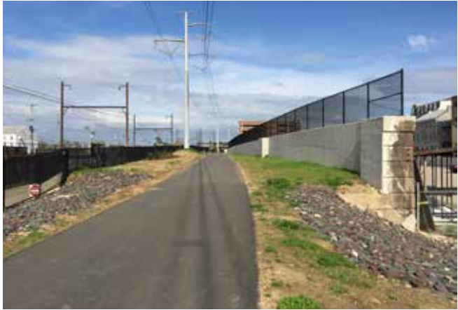
Photo 9: View facing east of the new retaining wall and asphalt pathway with new green space in the background.
