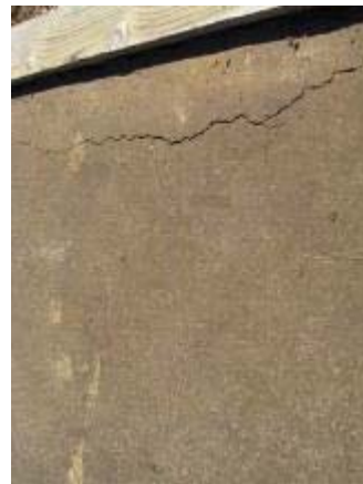
Photo 99 StaLok trail segment was noted for repairing itself. March 13, 2008.
