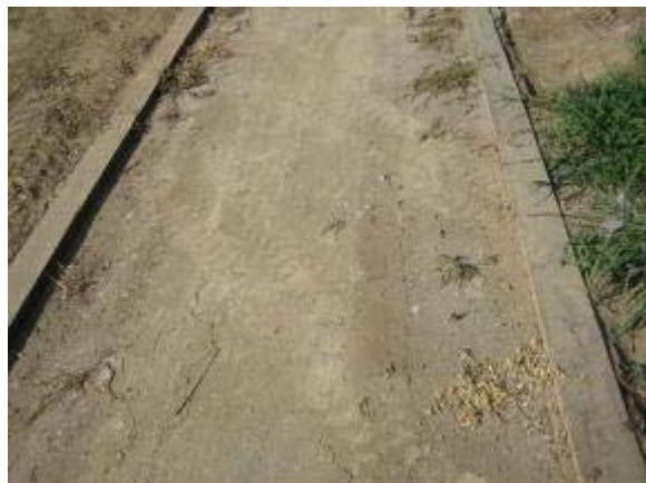
Photo 113 Polypavement trail segment after heavy rains remained cracked. August 9, 2007.
