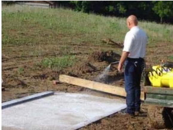
Photo 43 Soiltac Liquid Topical is applied to a base of 2 inch native soil, mixed with water and sprayed onto 4 inches of ¾ minus compacted limestone aggregate. June 27, 2007.
