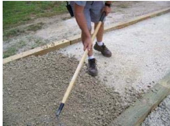
Photo 125 Three Quarter Inch Minus Limestone trail segment has second lift installed. August 3, 2007.
