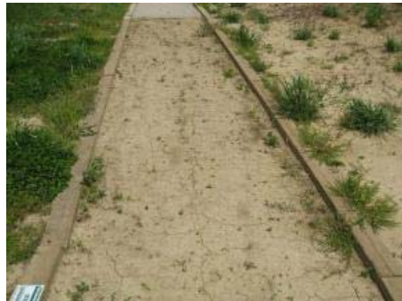
Photo 117 Polypavement trail segment shows cracks. May 6, 2008.
