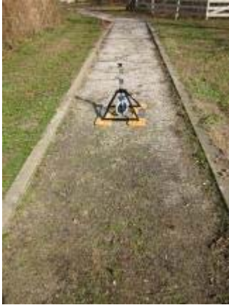
Photo 40 Soiltac Powder Mix-In showed only minor evidence of softening at the end of the study. November 2, 2011.
