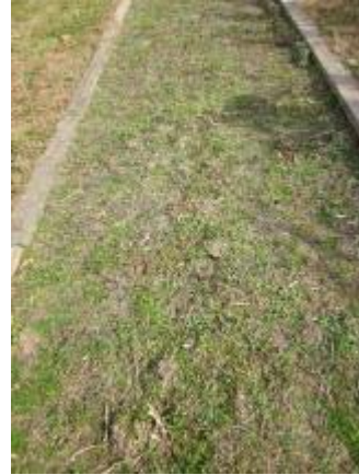
Photo 121 Polypavement trail segment overgrown with vegetation. November 2, 2011.
