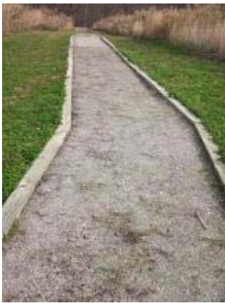
Photo 89 Stabilizer trail segment shows deterioration along timber edging. November 2, 2011.
