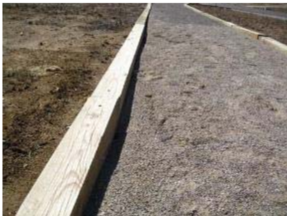
Photo 137 Quarter Inch Minus Limestone trail segment developed an erosion ditch. March 13, 2008.
