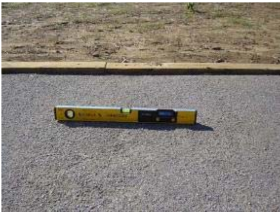
Photo 77 Stabilizer trail segment shows loose fines at top of surface. July 6, 2007.
