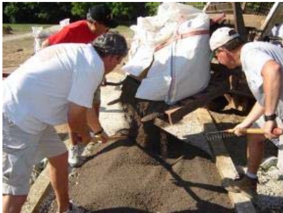
Photo 92 StaLok is applied at a 2 inch depth on top of the base. June 21, 2007.
