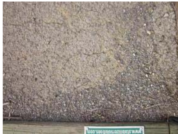
Photo 105 StaLok trail segment shows cracking next to timber edging. November 2, 2011.
