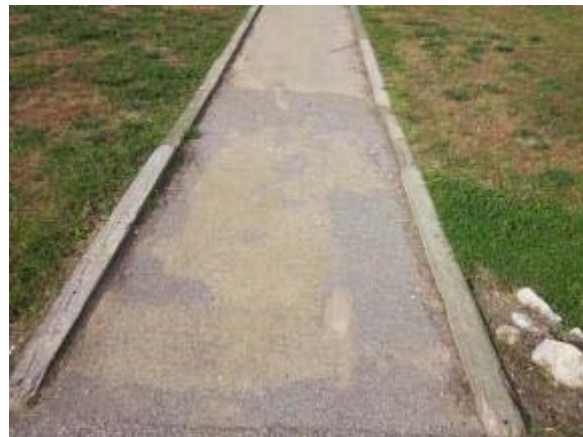
Photo 107 StaLok trail segment with pooling of water. November 2, 2011.
