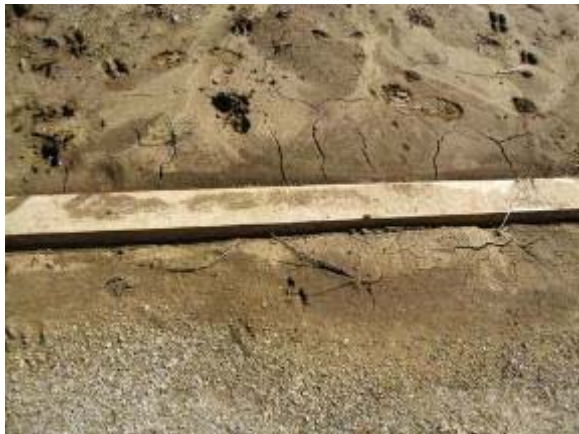
Photo 47 Soiltac Liquid Topical trail segment showed signs of runoff. March 13, 2008.
