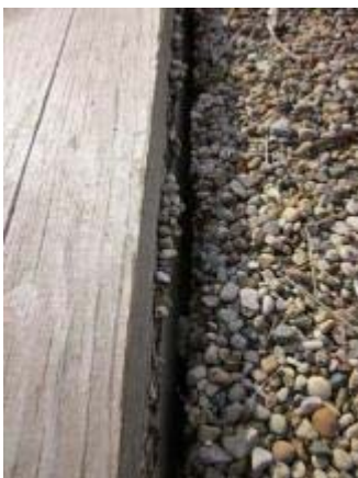
Photo 17 Klingstone surface has started to recede from timber edging. November 22, 2011.
