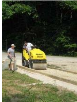
Photo 123 Three Quarter Inch Minus Limestone trail segment with 50 percent dust has first lift compacted. August 1, 2007.
