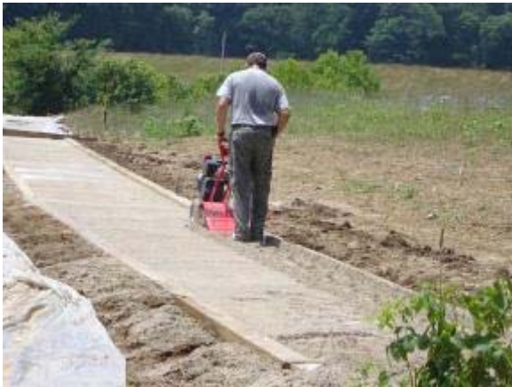
Photo 57 Soiltac Liquid Mix-In is then tilled into 4 inches of ¼ inch minus loose limestone aggregate. June 27, 2007.
