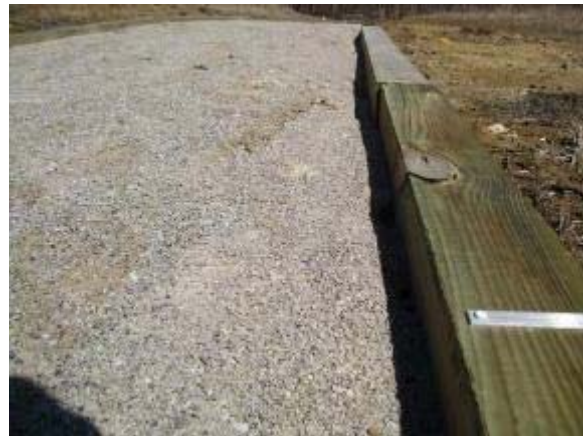
Photo 136 Quarter Inch Minus Limestone trail segment was loose under foot after heavy rainfall. March 13, 2008.
