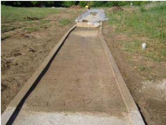
Photo 110 Polypavement trail segment started to show signs of cracking and softening after the first round of tests. July 6, 2007.
