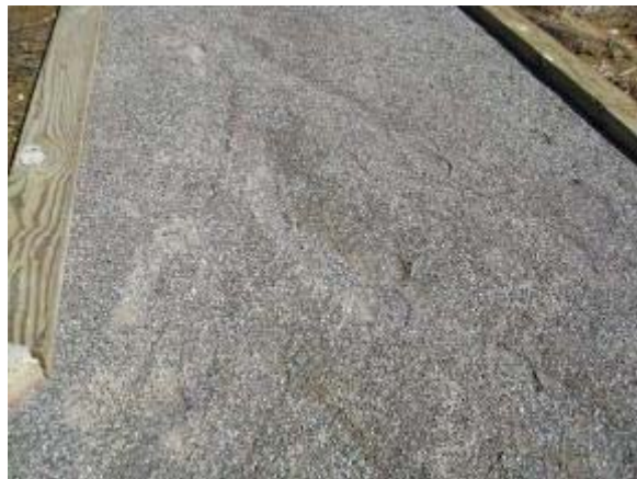
Photo 80 Stabilizer trail segment has runoff from heavy rainfall. March 13, 2008.
