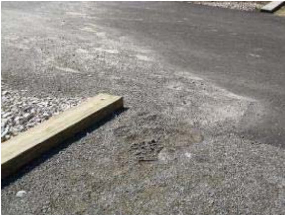
Photo 81 Stabilizer trail segment shows loose fines from heavy rainfall. March 13, 2008.
