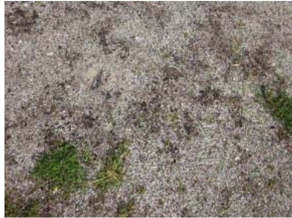
Photo 88 Stabilizer trail segment shows deterioration in middle of the trail. November 2, 2011.
