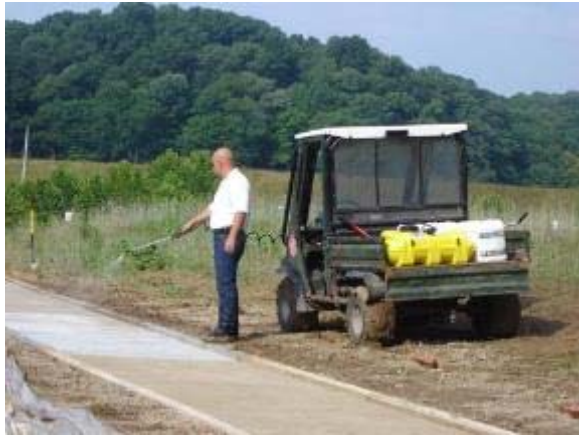
Photo 18 Soiltac Powder Topical is applied to a base of 2 inches of native soil and 4 inches of ¼ inch minus compacted limestone aggregate. June 27, 2007.
