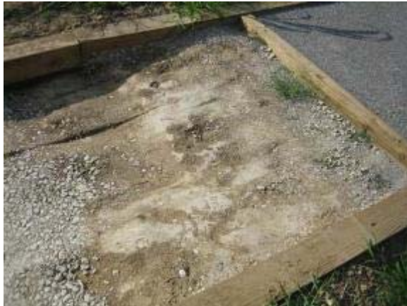
Photo 133 Quarter Inch Minus Limestone was installed in two rolled and compacted 3 inch lifts. August 9, 2007.
