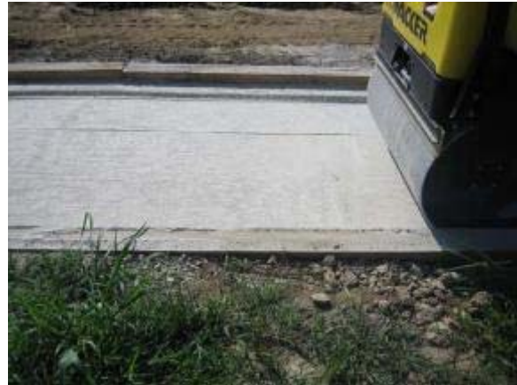
Photo 134 Quarter Inch Minus Limestone trail segment as second lift is rolled and compacted. August 9, 2007.
