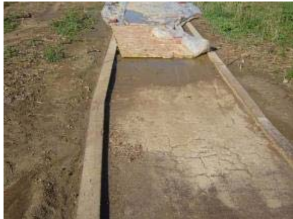
Photo 111 Polypavement trail segment started to show signs of cracking and softening after the first round of tests. July 6, 2007.
