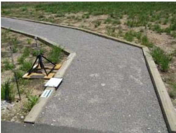
Photo 83 Stabilizer trail segment more than a year after installation. May 6, 2008.
