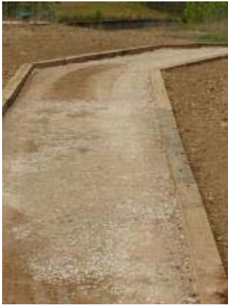
Photo 69 Stabilizer is applied to a base of 3 inches of compacted native soil. June 19, 2007.
