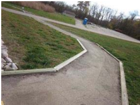
Photo 106 StaLok trail segment had some pooling of water at lower points of the surface. November 2, 2011.
