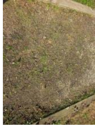
Photo 41 Soiltac Powder Mix-In trail segment with water crossing would soften and then return to natural surface state. November 2, 2011.
