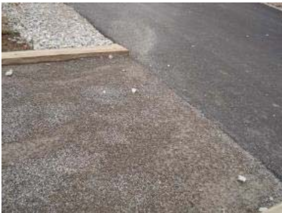
Photo 79 Stabilizer trail segment shows loose fines at top of surface. October 19, 2007.
