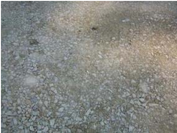
Photo 124 Three Quarter Inch Minus Limestone with 50 percent dust after first lift is compacted. August 1, 2007.
