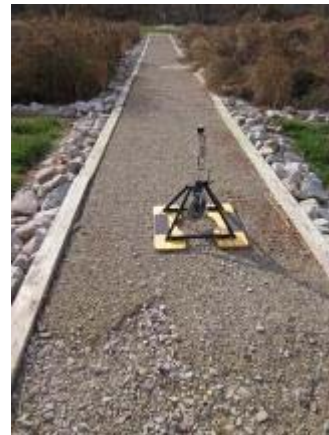
Photo 16 Klingstone at beginning of trail segment has started to wash out. November 22, 2011.
