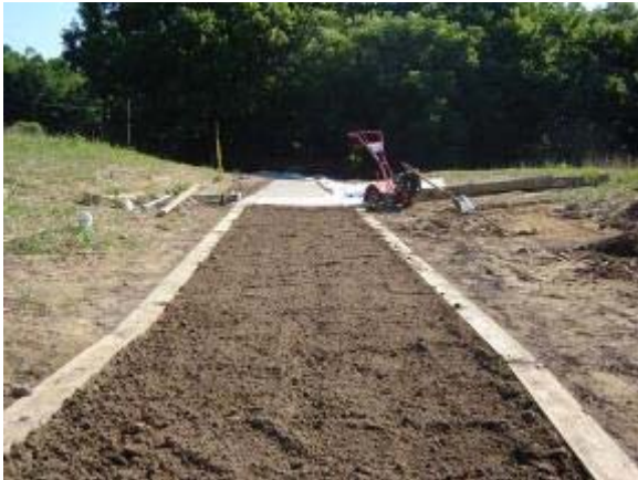
Photo 108 Polypavement is applied to a base of compacted native soils and mixed into an additional 2 inches of tilled soil. July 3, 2007.
