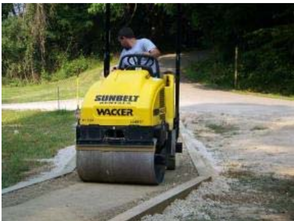
Photo 126 Three Quarter Inch Minus Limestone trail segment has second lift compacted. August 3, 2007.
