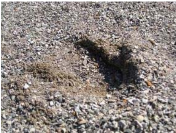
Photo 85 Stabilizer trail segment shows gullies created in surface from runoff. March 17, 2009.
