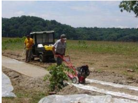
Photo 56 Soiltac Liquid Mix-In is then tilled into 4 inches of ¼ inch minus loose limestone aggregate. June 27, 2007.
