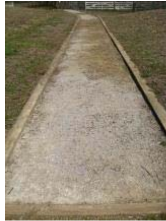
Photo 50 Soiltac Liquid Topical trail segment remained soft where water had pooled. March 17, 2009.
