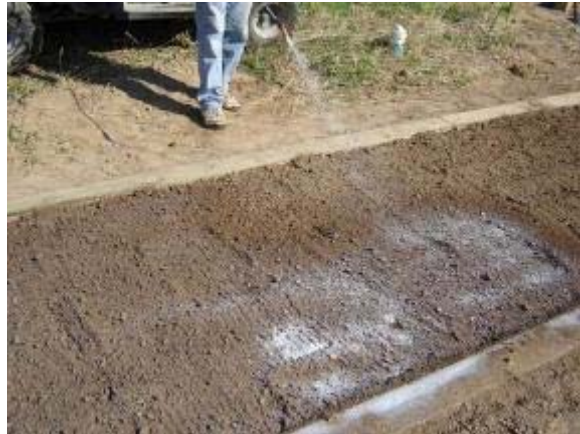
Photo 109 Polypavement is applied to a base of compacted native soils and mixed into an additional 2 inches of tilled soil. July 3, 2007.
