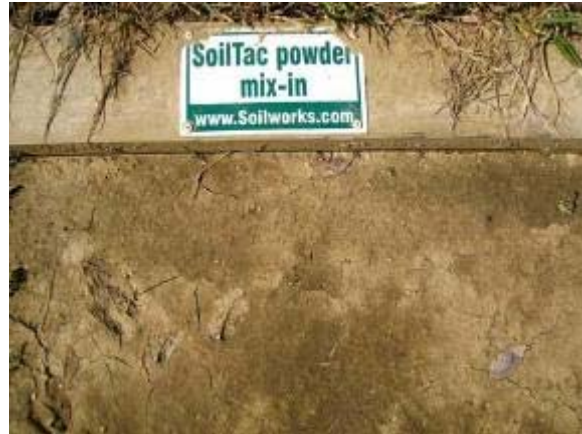
Photo 35 Soiltac Powder Mix-In almost a year after installation. March 13, 2008.
