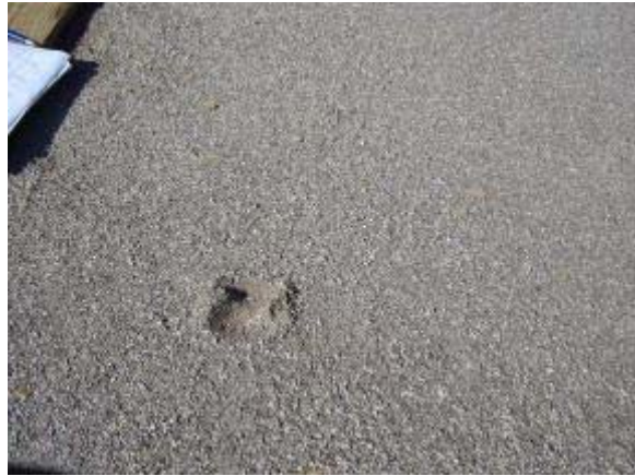
Photo 76 Stabilizer surface shows an indentation from the surface testing. July 6, 2007.
