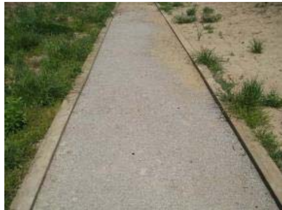
Photo 48 Soiltac Liquid Topical trail segment remained soft where water had pooled. May 6, 2008.
