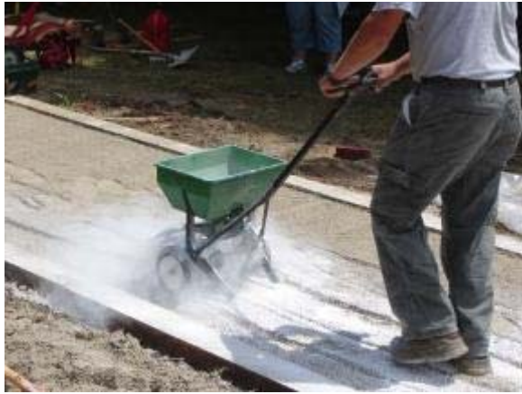
Photo 28 Soiltac Powder Mix-In is applied to a base of 2 inches of native soil. June 27, 2007
