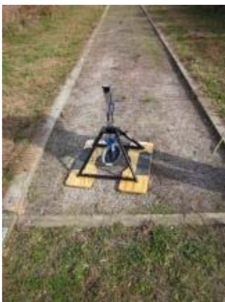
Photo 53 Soiltac Liquid Topical trail segment remained soft through the final testing. November 2, 2011.
