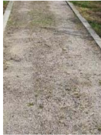
Photo 146 Three Quarter Inch Minus Base and Quarter Inch Minus Top Limestone trail segment became firm and stable under foot more quickly than the ¼ inch surface. November 2, 2011.
