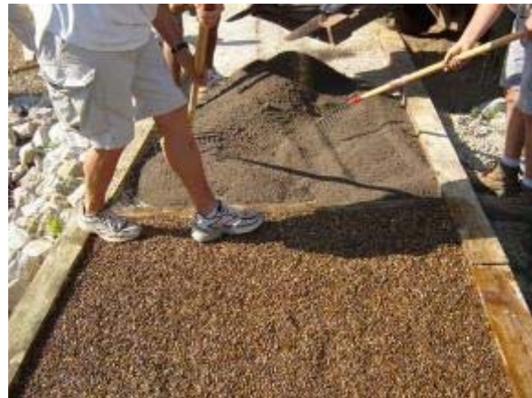
Photo 93 StaLok is applied at a 2 inch depth on top of the base. June 21, 2007.
