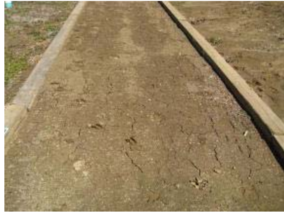
Photo 115 Polypavement trail segment would dry with cracks and heaving after heavy rail. March 13, 2008.
