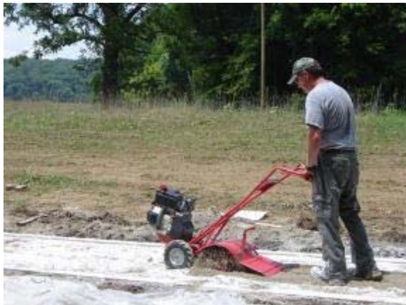
Photo 30 Soiltac Powder Mix-In is tilled into the 2 inch base of native soil. June 27, 2007.
