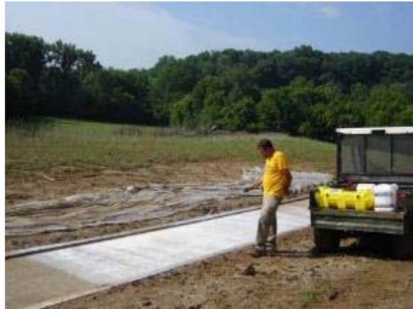
Photo 19 Soiltac Powder Topical is applied to a base of 2 inches of native soil and 4 inches of ¼ inch minus compacted limestone aggregate. June 27, 2007.
