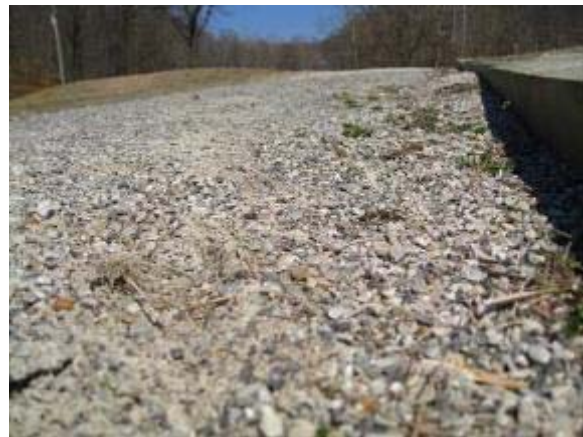
Photo 86 Stabilizer trail segment shows deterioration from runoff along timber edging. March 17, 2009.
