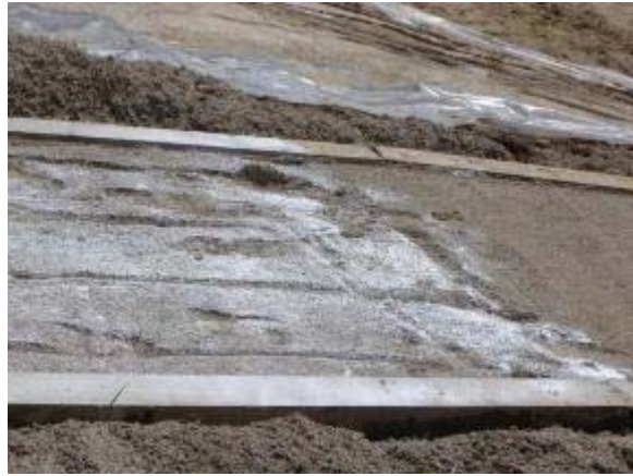
Photo 29 Soiltac Powder Mix-In is applied to a base of 2 inches of native soil. June 27, 2007.
