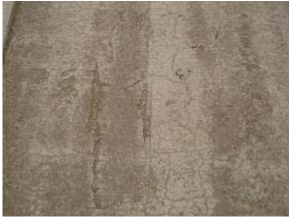
Photo 114 Polypavement trail segment with cracks and heaving along width of trail. October 19, 2007.
