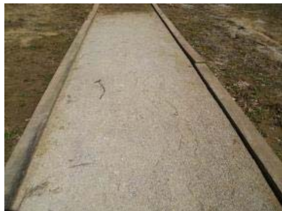
Photo 64 Soiltac Liquid Mix-In trail segment was only slightly soft under foot, showing footprint indentations. March 13, 2008.
