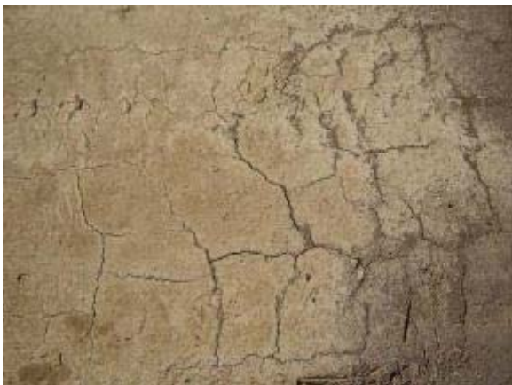
Photo 112 Polypavement trail segment shows cracking. July 6, 2007.
