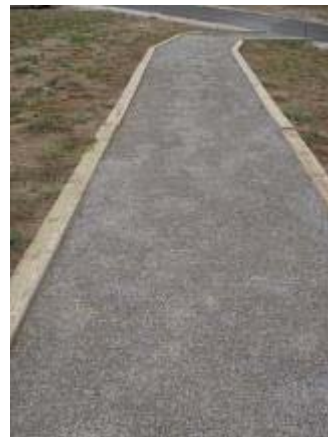
Photo 78 Stabilizer trail segment shows loose fines at top of surface. October 19, 2007.
