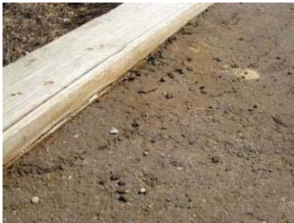
Photo 98 StaLok trail surface had a pattern of wear and repairing itself. March 13, 2008.
