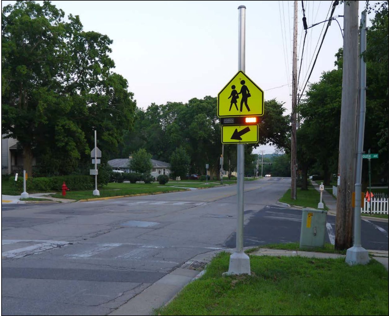
Figure 3.7: Rectangular Rapid-Flashing Beacon
