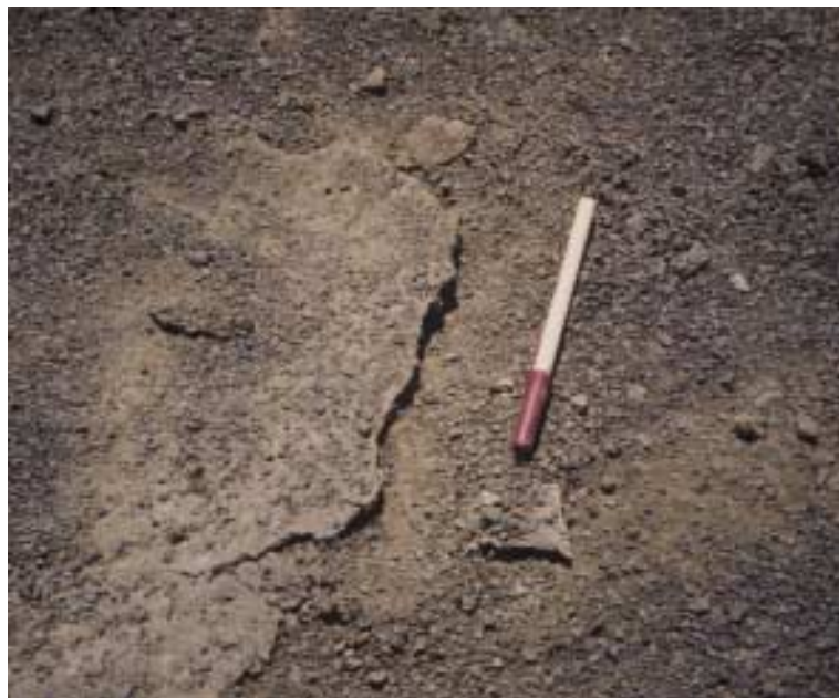
Figure 5. Crack that developed in trail after second winter.
