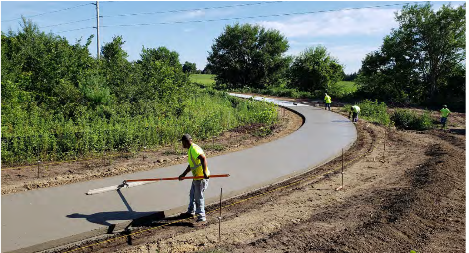
The Solon to Ely section of the Hoover Nature Trail under construction | Photo courtesy Johnson County Conservation Board
